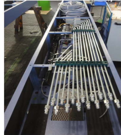
Image 11: The supply lines for hydraulics, pneumatics and lubrication are accommodated in the installation profiles.
